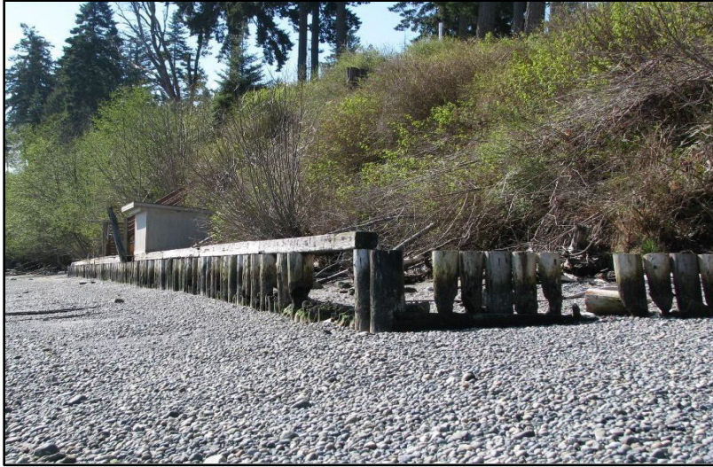
Figure 27: Removal Credits for Old Creosote Bulkhead: Removal credit applied for creosote, not for remnants of bulkhead. Picture by and with permission from Doris Small, WDFW.
